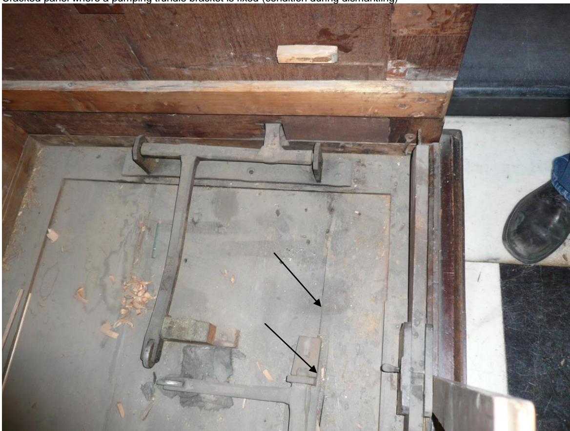
Cracked panel where a pumping trundle bracket is fixed (condition during dismantling)
