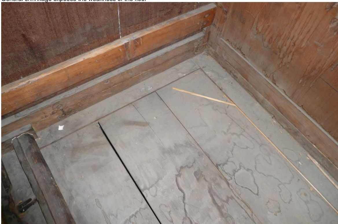
General shrinkage exposes the weakness of the floor
